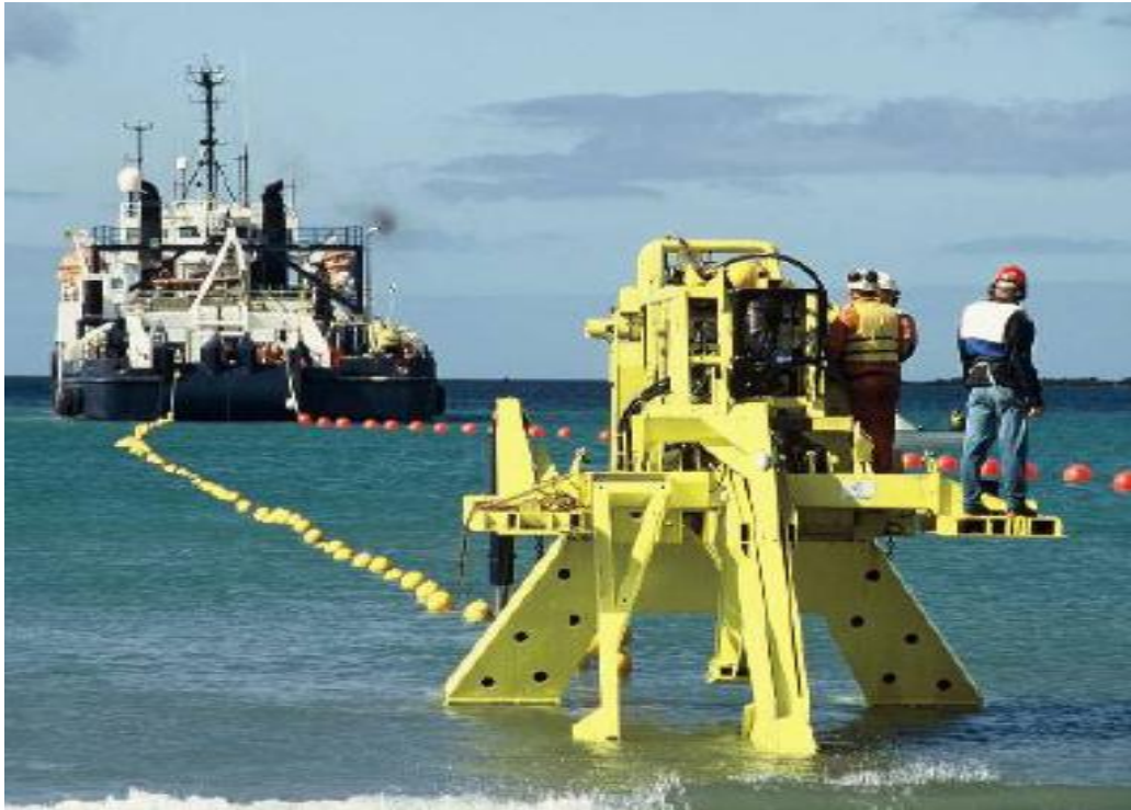
Figure 5. Sea plow and cable ship about to bury submarine cable (from ISPC 2009)
